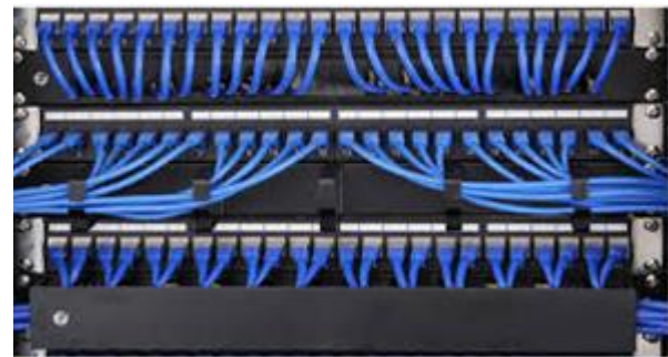
Fig. 2. Termination of Cables on the Patch Panel
