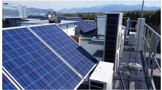
Fig. 3.2. Photo of a partially shielded SV60-255 photovoltaic panel.
