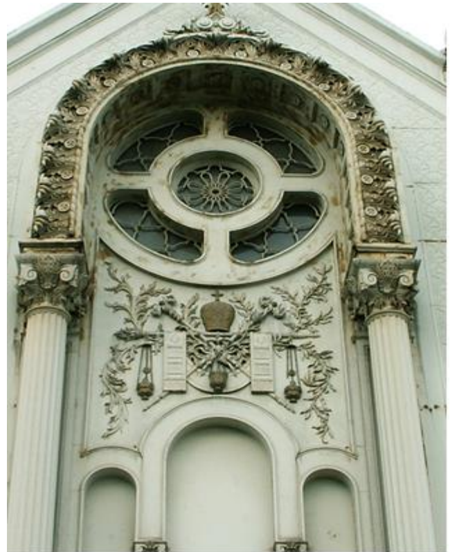
Figure 10: Detail from the south façade of the transept and Symbols on the transept walls
