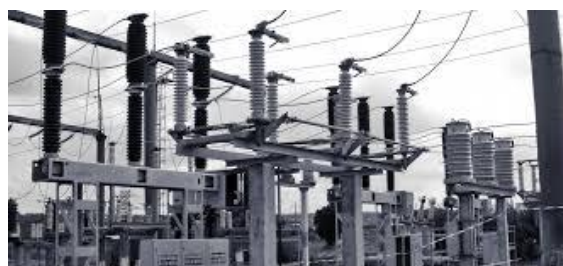
Fig. 1. A typical 132/20 kV high voltage substation (outdoor switchyard).
